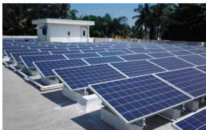
375 kWp Roof Top Solar PV Grid connect Power plant – AUMA India Building Roof Top Solar Plant: A new paradigm for AUMA India’s self-generation for captive consumption
