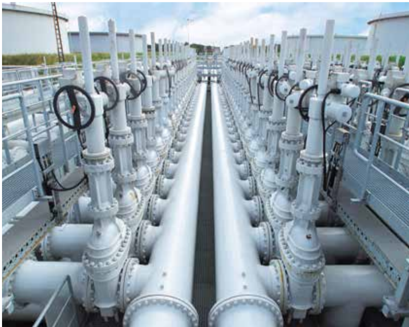
AUMA Actuators – Typical application @ Marketing Terminal complex
